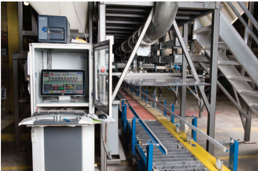
The weighing and batching system’s PLC controller controls and monitors the entire batching operation, allowing an operator to easily input and access the various recipes.
