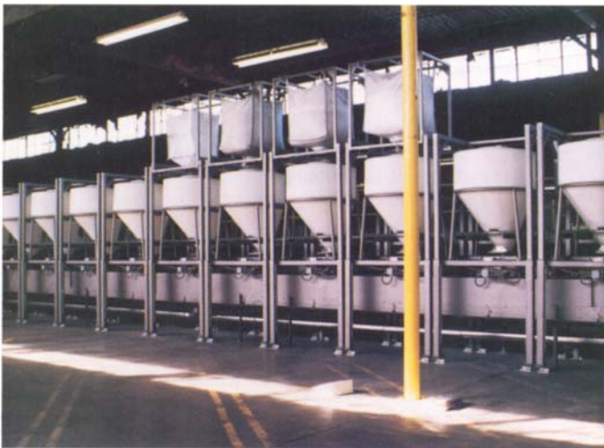
The batching system allows the refractory producer to receive and handle many different ingredients and automate the batching process.
