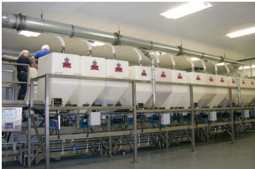
Operators on the system’s walkway platform, mounted directly above the weighbelt conveyors, have easy access to the dispensers for inspection and refill.
